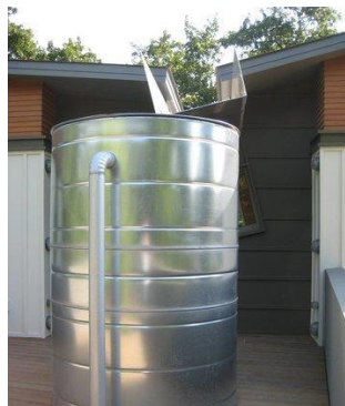
Photo 15: Commercial Rain Barrel Example
